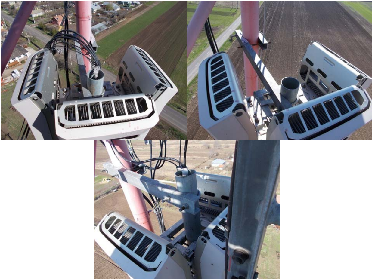
Swap existing 01B3 RRU's with new 2217/2219 RRU's
