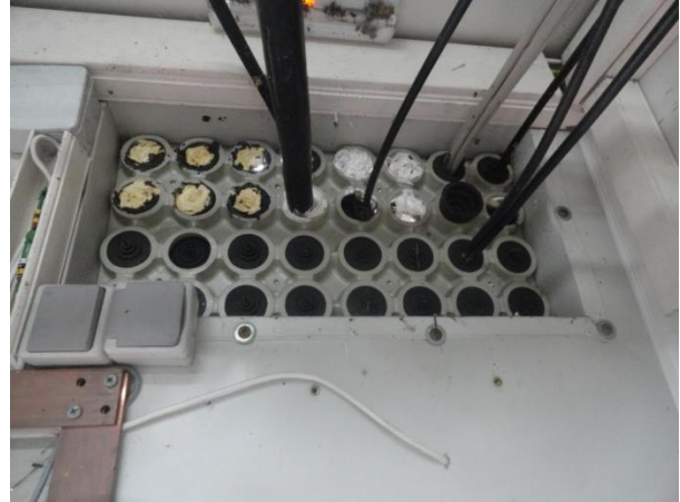
Intrare cabluri in shelter la interior
